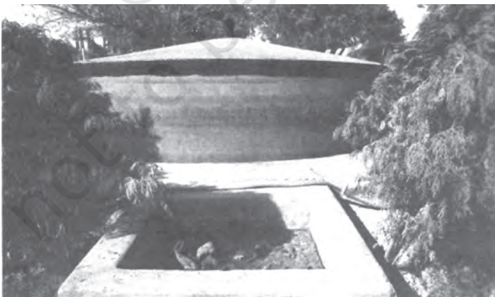
Fig. 7.4 Gobar Gas Plant uses cattle dung to produce energy
